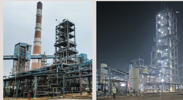
Overall View of the Methanol Synthesis Demonstration Plant Installed in the Power Plant
