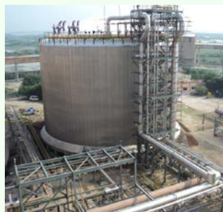
An ammonia storage tank (from a past project of Toyo-India)
