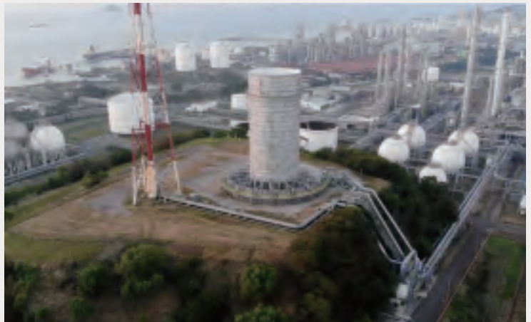
The enclosed ground flare system
