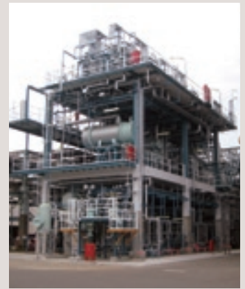
Completed ETBE plant
