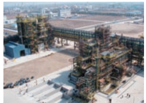
Siloxane project for Dow Corning Corporation in China
