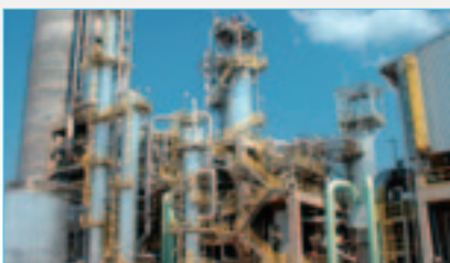
1,725 t/d ACES21® urea plant of PT. Pupuk Kujang (Indonesia)
