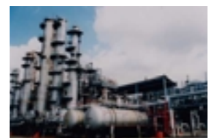
Existing VCM plant
