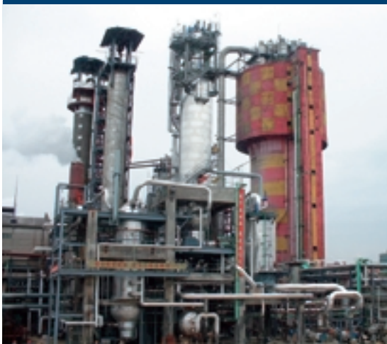
ACES 21® Urea Plant Sichuan Chemical Works (Group) Ltd., Sichuan, China
