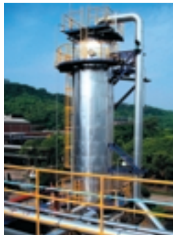
MRF-Z ® Reactor at No.2 Methanol Plant in SINOPEC Sichuan Vinylon Works
