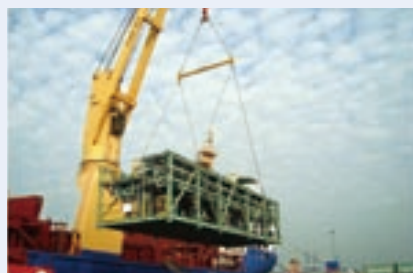
Module of Micro-GTL demonstration plant being loaded on ship in Thailand bound for Brazil
