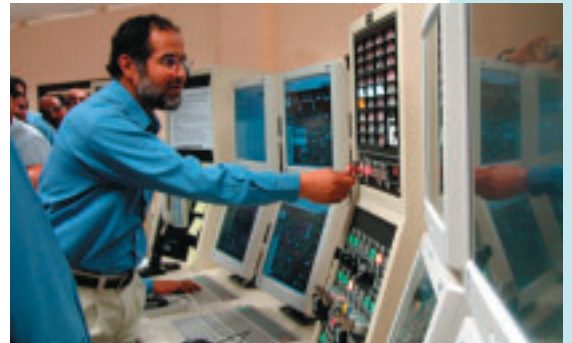
Start-up of 2nd EO / EG plant of Jubail United Petrochemical Company in Saudi Arabia
